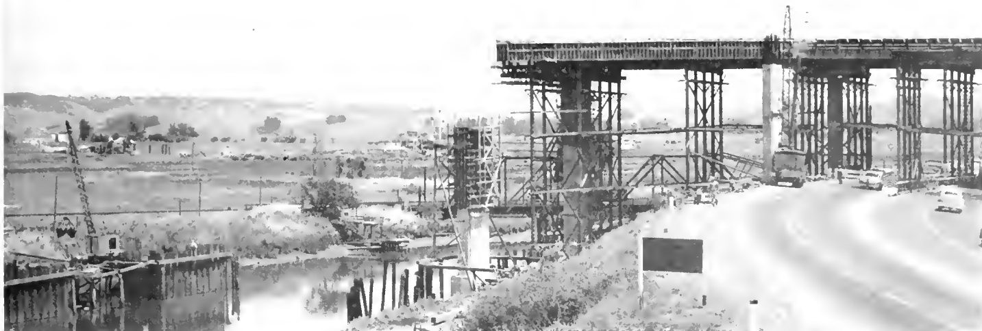
Looking easterly at Petaluma Creek Bridge and Overhead during construction. Present Redwood Highway (US 101) carried through construction with very little inconvenience to traffic.
